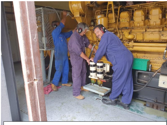
Dougie, Robin and Raymond preparing to disconnect the alternator from the engine on No.1 generator to remove the flywheel and replace the crankshaft oil seal. Then replace the coupling.
