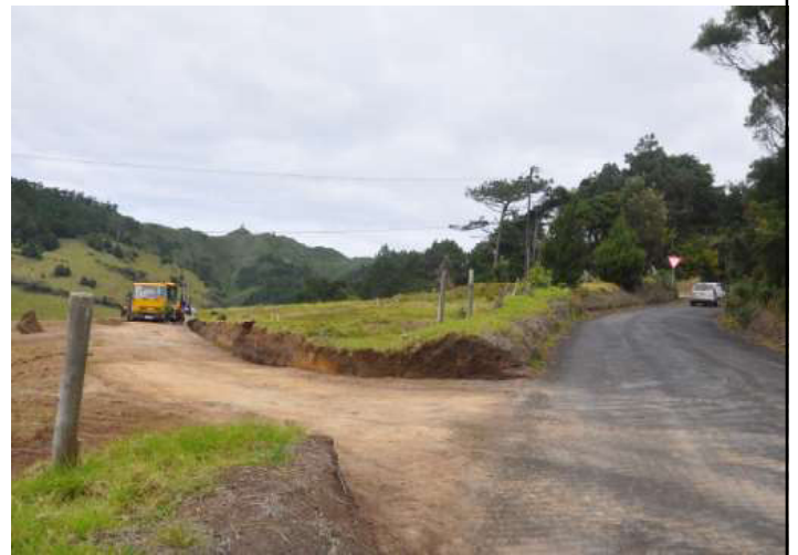
Conversion of part of a cow field into a cemetery just across the road from the Dungeon Cemetery; the photo shows the flattest areas in the cemetery extension, the land falls further to the south and east.
