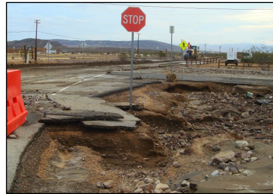
Flooding in the cantonment area at Fort Irwin, CA in August 2013 (US Army Photo)
