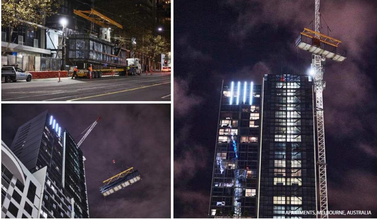
Figure 5 Modules being transported on-site and being craned into position for final assembly. Final constructed building stands at 44 floors.
