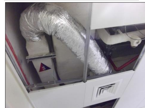
Figure 1: Common examples of design decisions or oversights that can impact the performance gap in a building.
