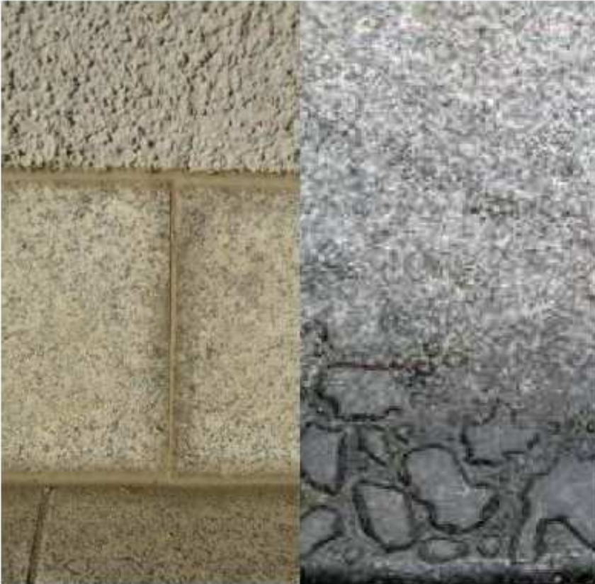
Staining of natural stone
