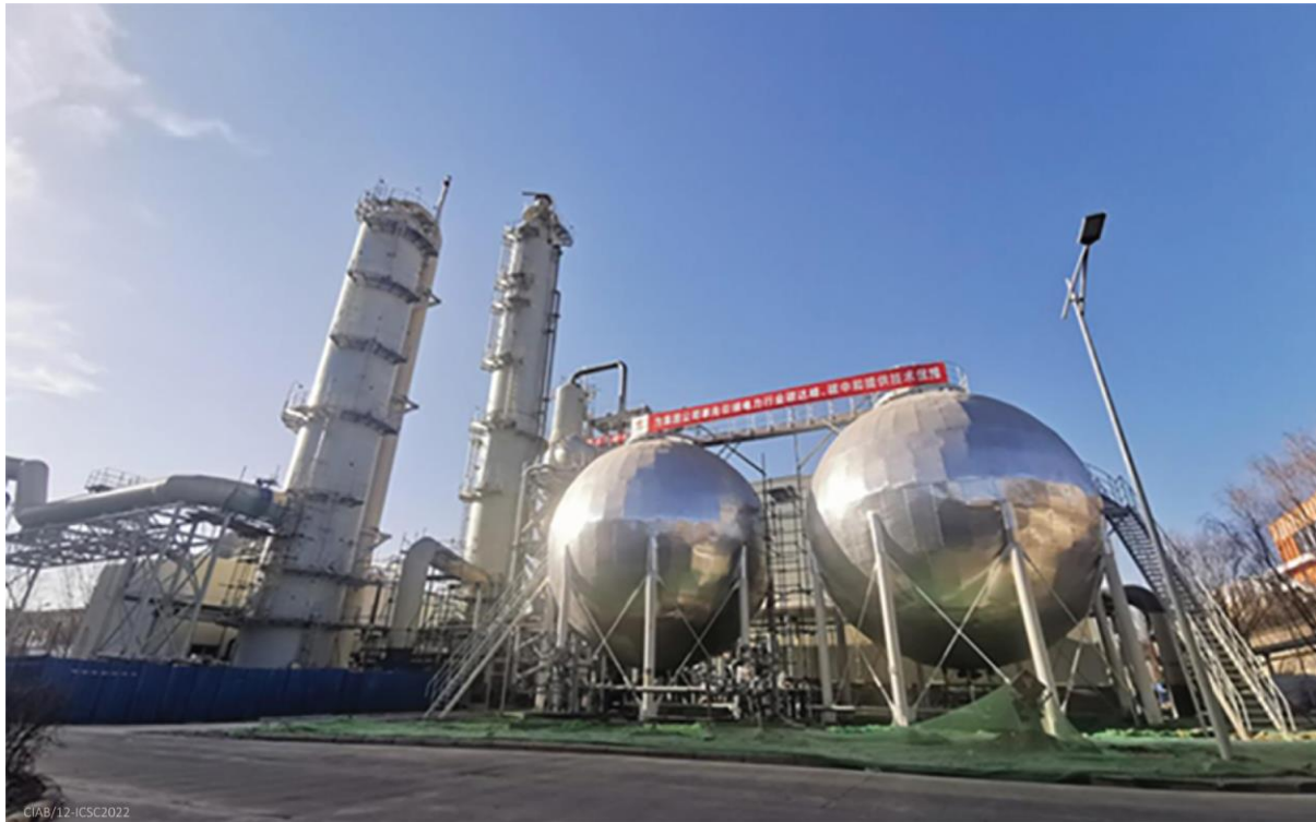
Figure 12 Jinjie Energy's 0.15 MtCO 2 /y CCUS facility (SASAC, 2021)
