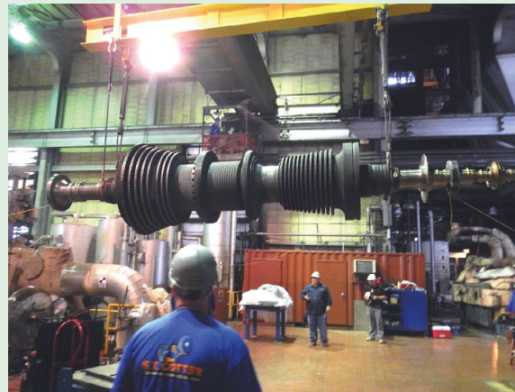
Figure 11. FutureGen 2.0 Turbine Rotor (photo credit, FutureGen Alliance)
