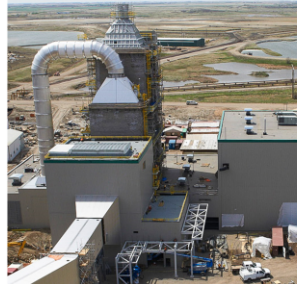
CCS at Boundary Dam 3 Power Station
