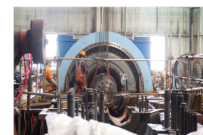
Inside the BD3 Power Generator during scheduled maintenance
