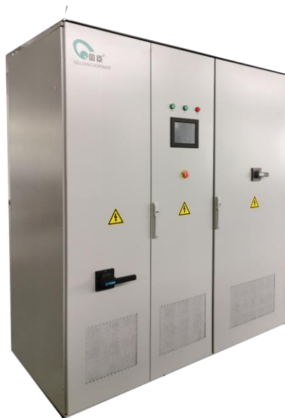
Grid connected inverter
