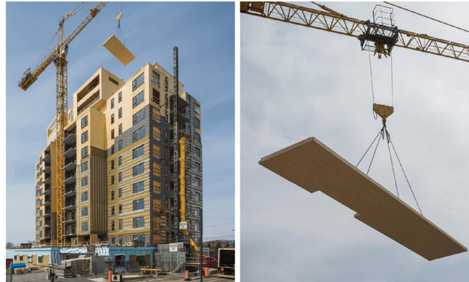
Mass timber panels save construction time. The wooden structure for the Origine project was erected in just four months. It was estimated that about a 25% savings in total project construction time resulted from selecting the mass timber panel structural system. (Cecobois)
