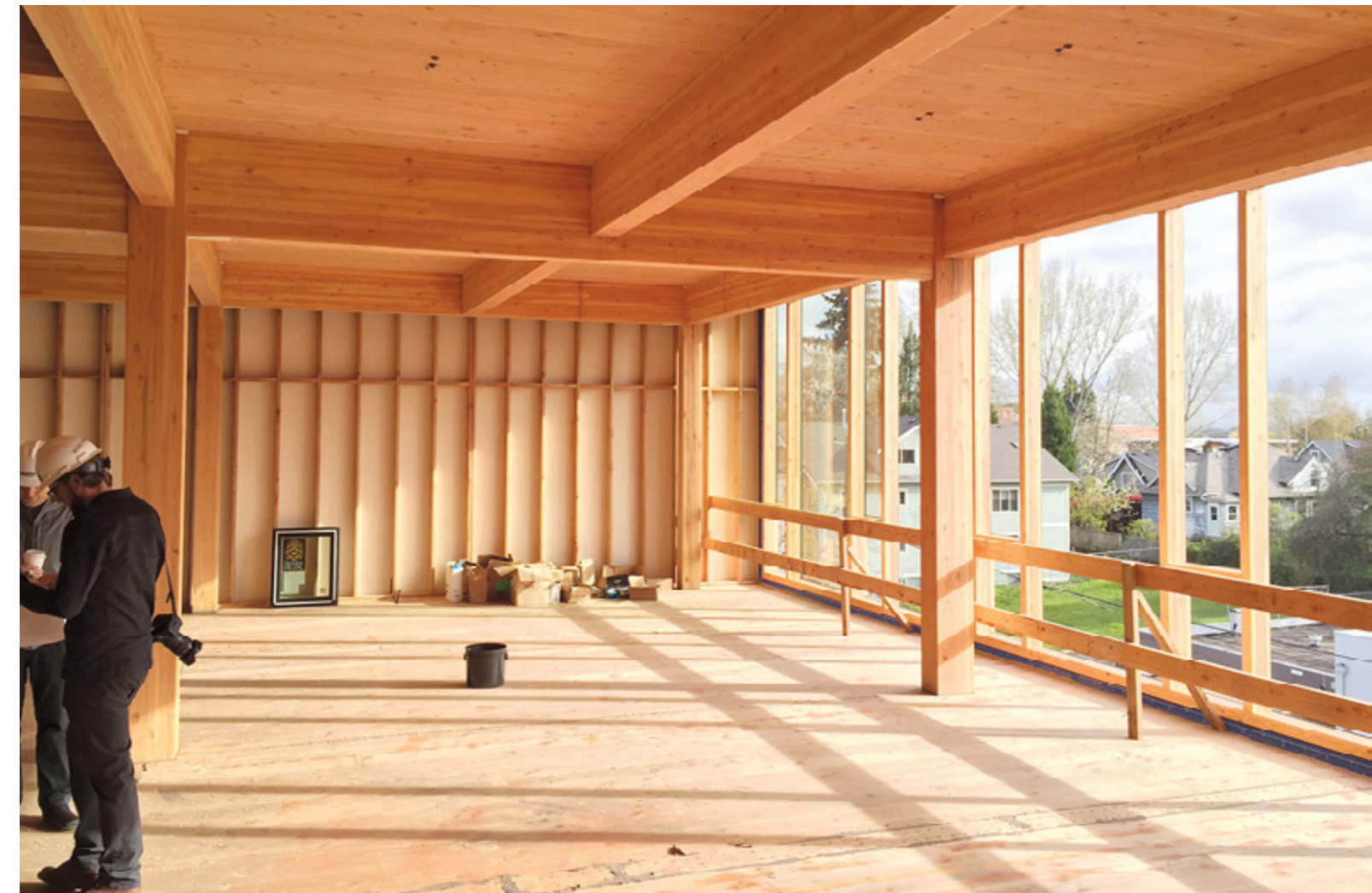
Post and beam mass timber evokes depth and warmth. Modern buildings with flat painted ceilings are not as expressive and inviting as exposed wood columns, beams and decking. (Albina Yard, Portland, Oregon by LEVER Architecture.)
