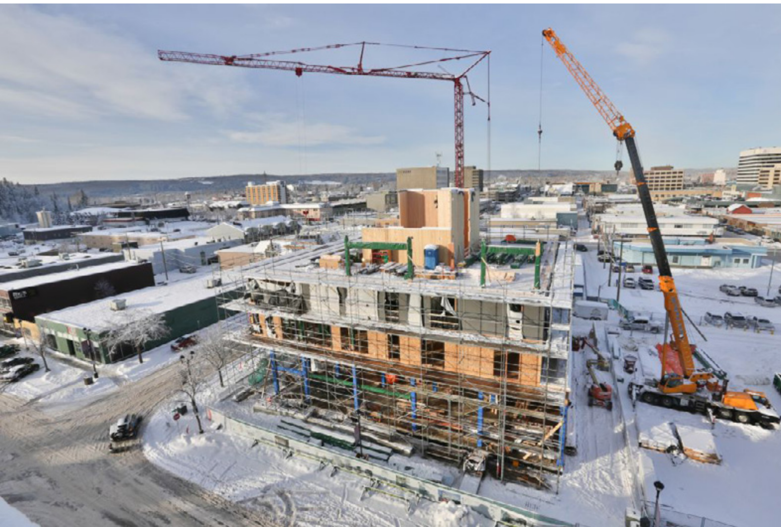
Minimize the number and duration of hoisting equipment rentals. This construction site indicates a variety of cranes, lifts and scaffolding. A generous staging area beside the building and access behind the building allow cranes to work around the entire building without interference. Each project is different and considerable construction experience is needed to optimize the mix of hoisting equipment to efficiently execute the work. (Construction Canada)
