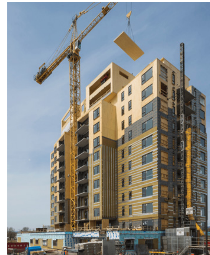
Conventional enclosure over multi-storey, loadbearing mass timber panels in balloon frame configuration. Water resistive air barrier membrane, mineral wool insulation between girts and cladding are applied after the panels are erected to complete the structure. (L'Origine – Nordic Structures)
