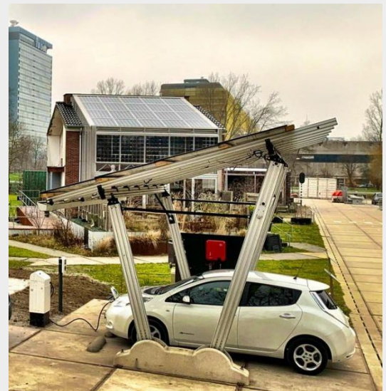
Figure 13: Dutch EV charging station at the Green Village
