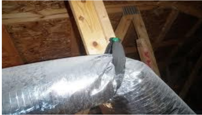
Improper ducting installations
