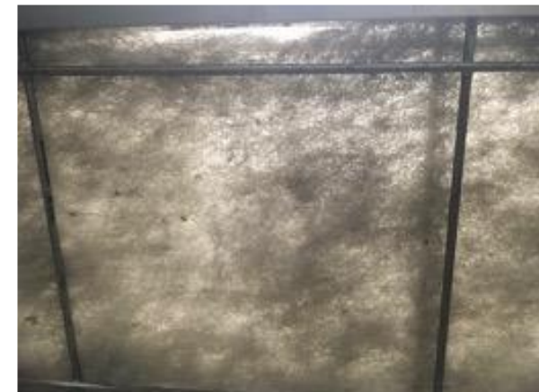
Poor filtration systems
