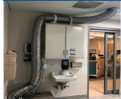
PHOTO 2 Don't use the existing return air duct system for exhaust (Lesson 6).
