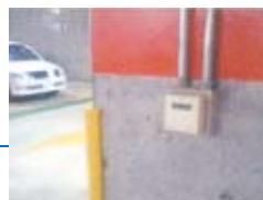
Carbon monoxide (CO) meter for controlling ventilation based on CO concentration level at car parking space
