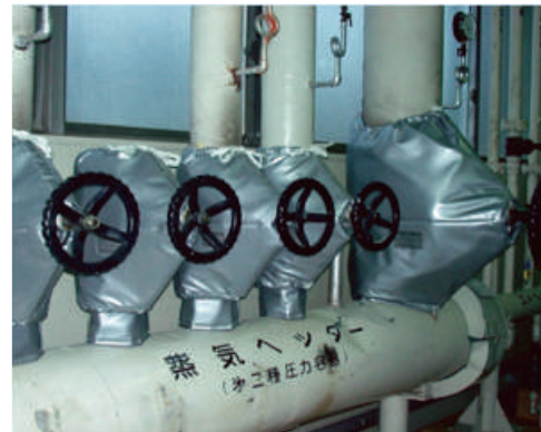
Fig. 2 Example of thermal insulation of steam header valve
