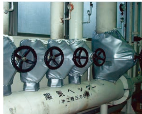
Fig. 2 Example of thermal insulation of steam header valve
