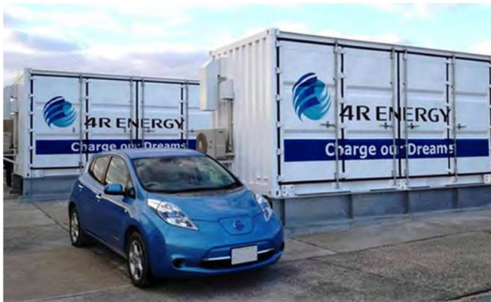
4R ENERGY BATTERY STORAGE SYSTEMS
