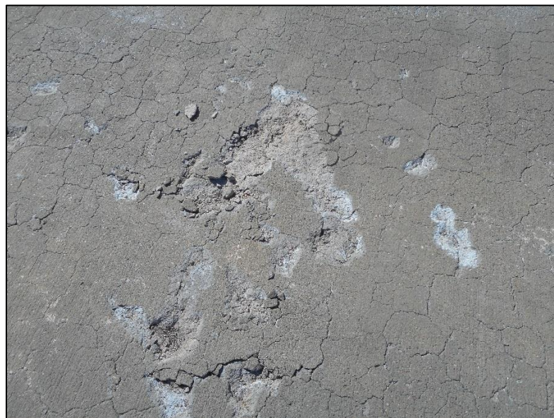
Figure 2-3. Spalling at Surface of Cal Pads
