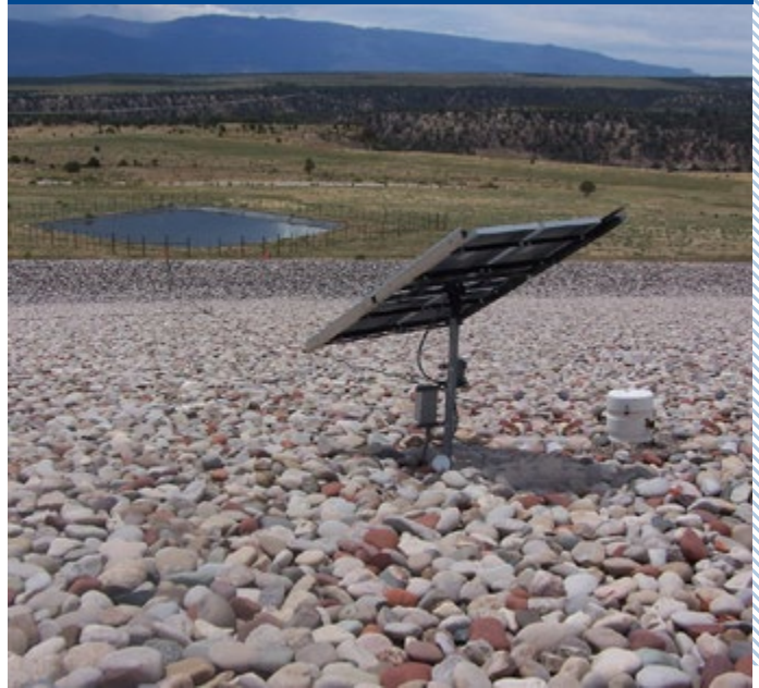
LM upgraded the solar power systems at the Rifle, Colorado, Disposal Site to increase system efficiencies during winter operations.
