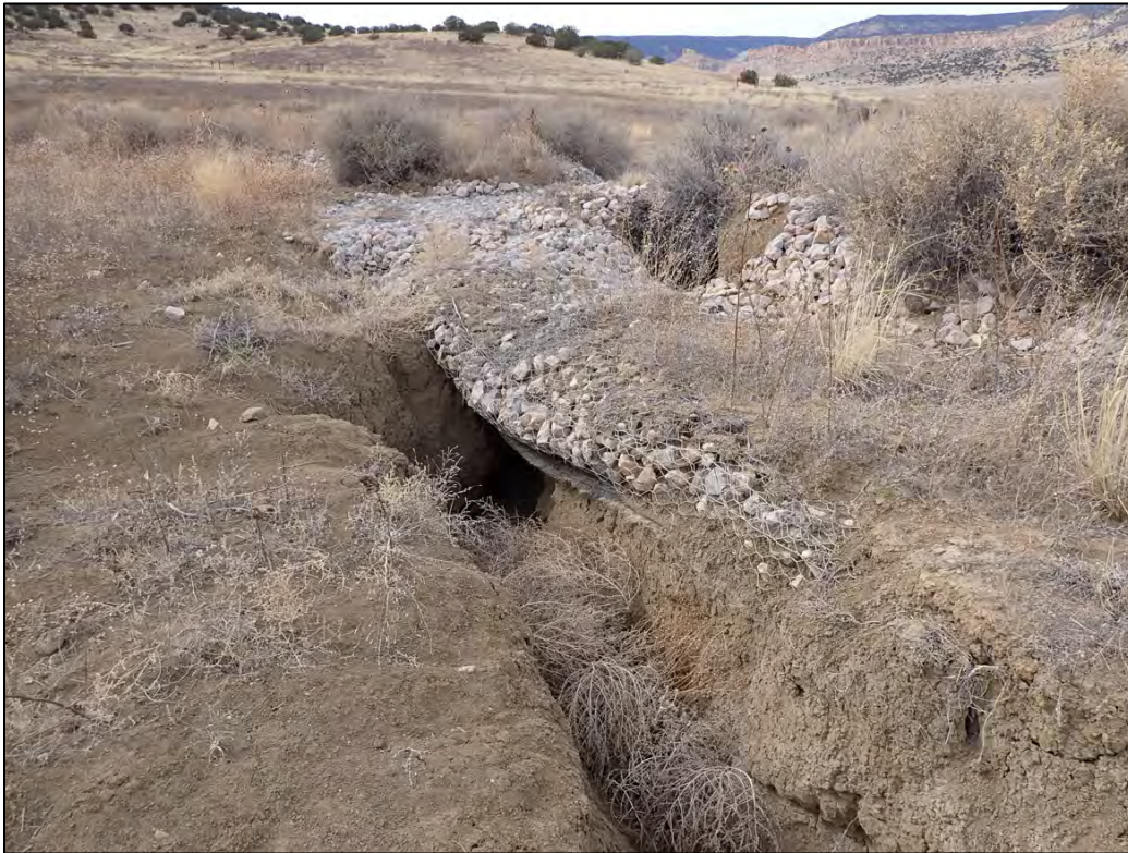
PL-17. Erosion at Structure A
