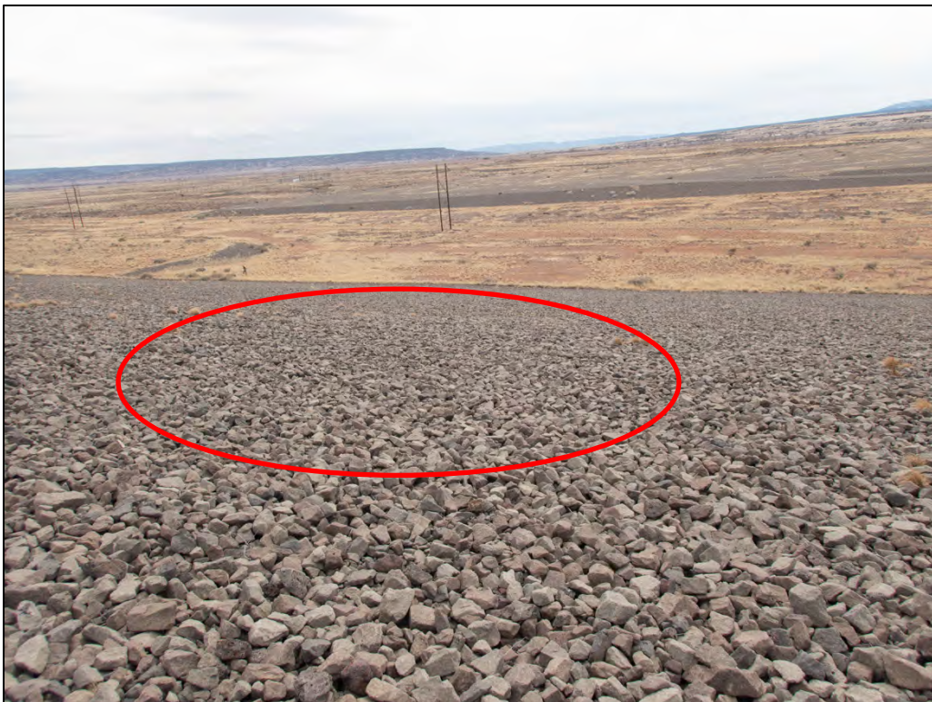
PL-14. Potential Depression Area on Main Tailings Disposal Cell Southwest Side Slope
