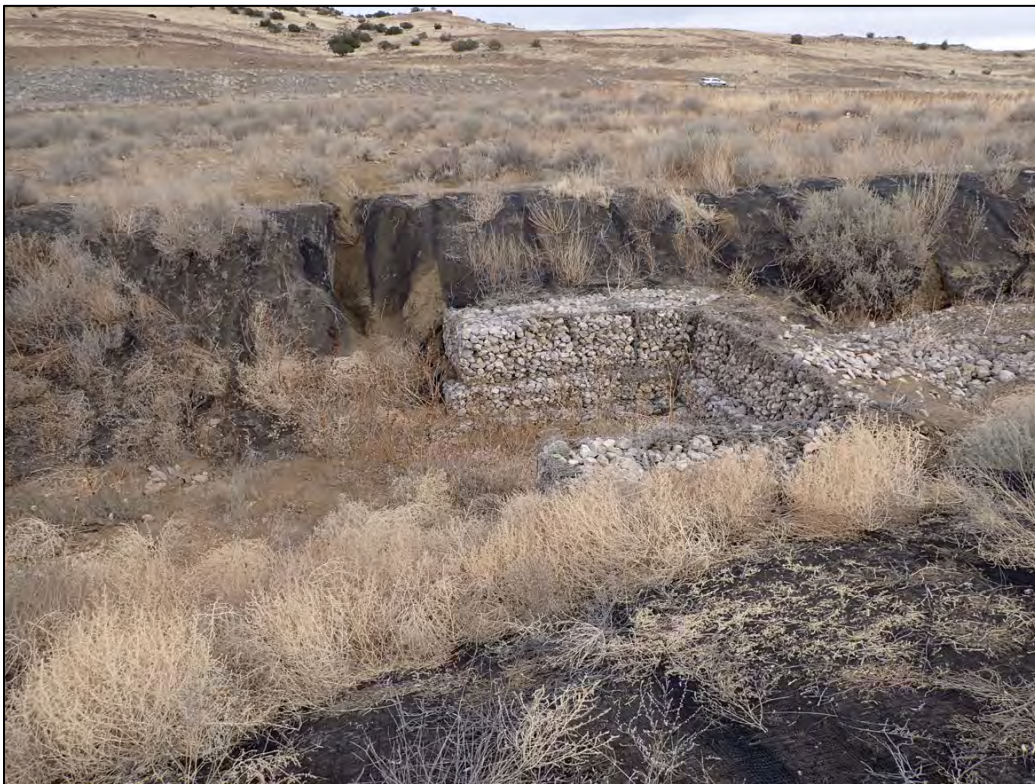
PL-18. Erosion at Structure A Along Second Block Structure
