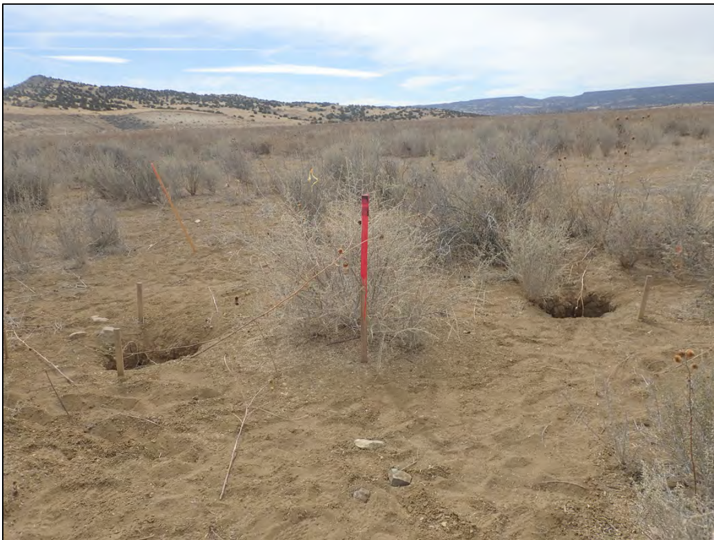
PL-10. Degradation Feature E-004 on Disposal Cell Top Slope
