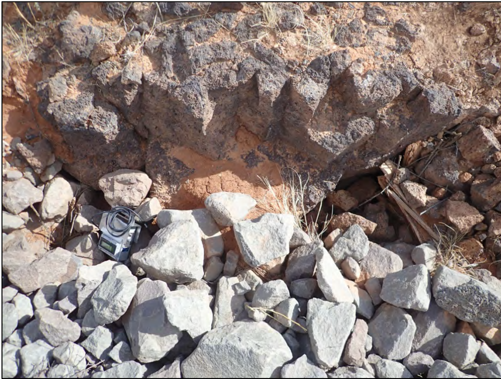
PL-23. East Dump Minor Erosion Area
