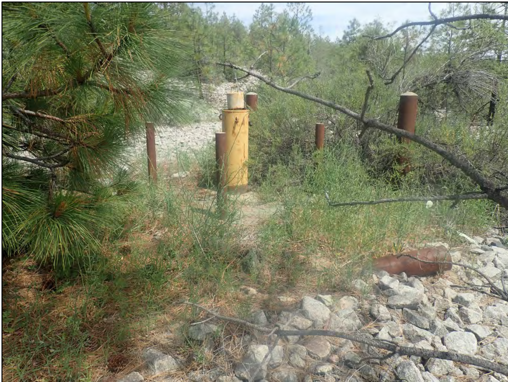
PL-4. Monitoring Well MW-4 with Damaged Bollard
