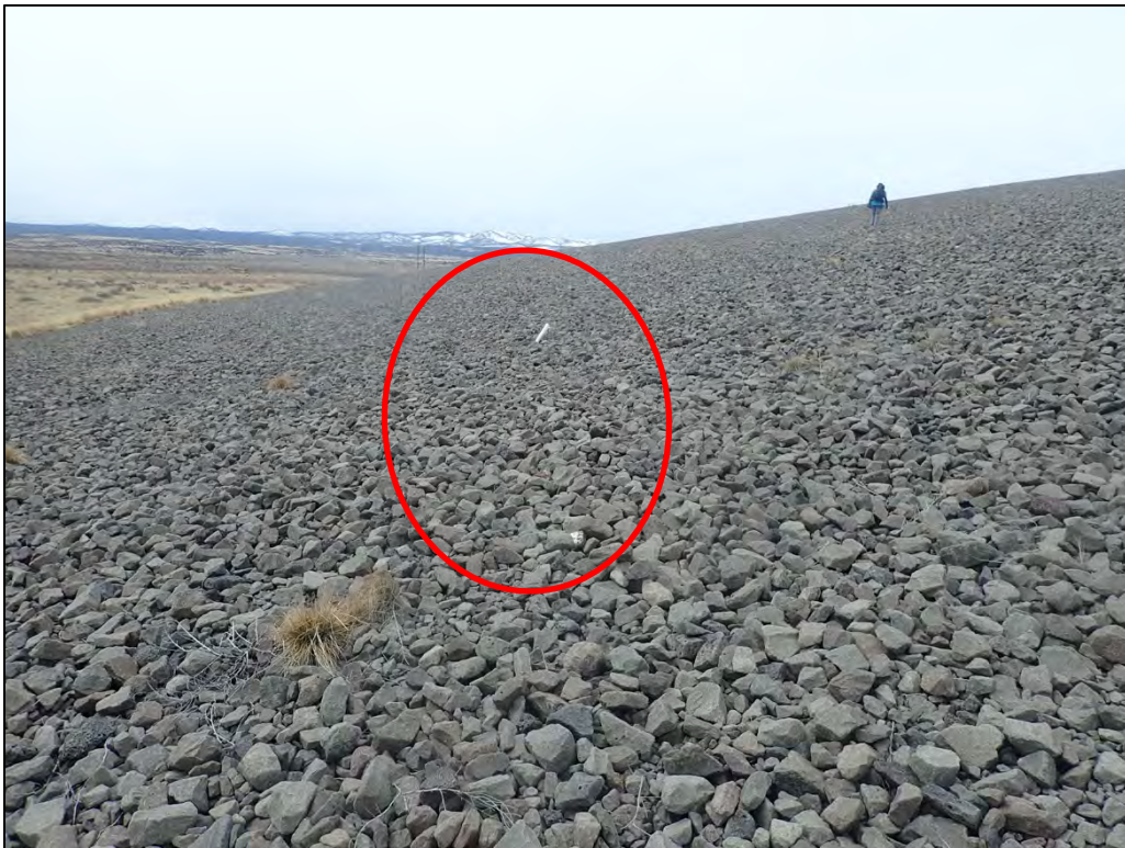
PL-16. Minor Depression on Main Tailings Disposal Cell South Side Slope
