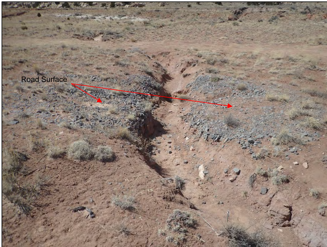
PL-1. Erosion of Site Road Along Northwestern Corner
