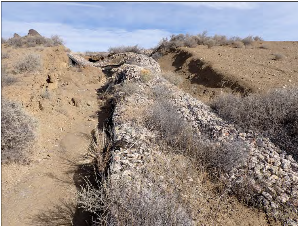
PL-16. Gully Erosion at Erosion Control Structure G
