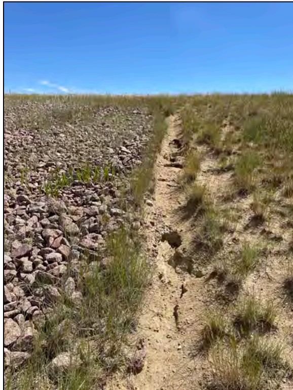
PL-8. Erosion Caused by Animal Trail South of Upper Riprap Slope
