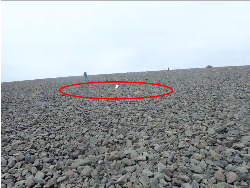
PL-15. Minor Depression on Main Tailings Disposal Cell South Side Slope
