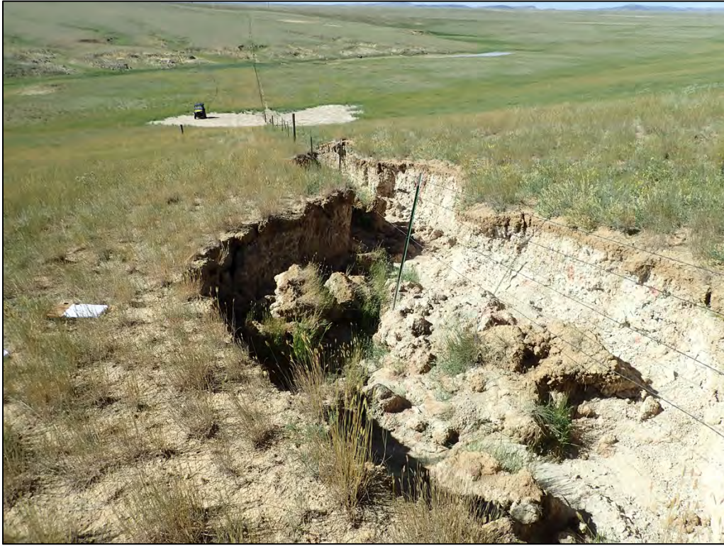
PL-1. Arroyo Under Fence on Lower Reclaimed Slopes
