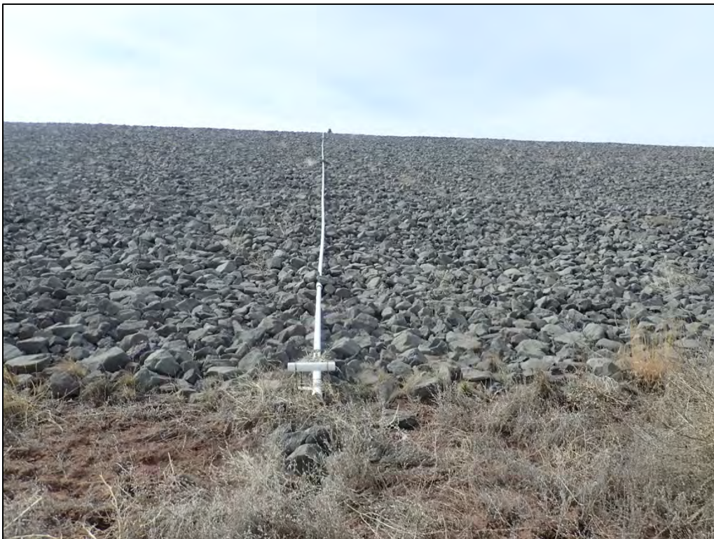
PL-12. Siphon Outlet on Main Tailings Disposal Cell North Side Slope
