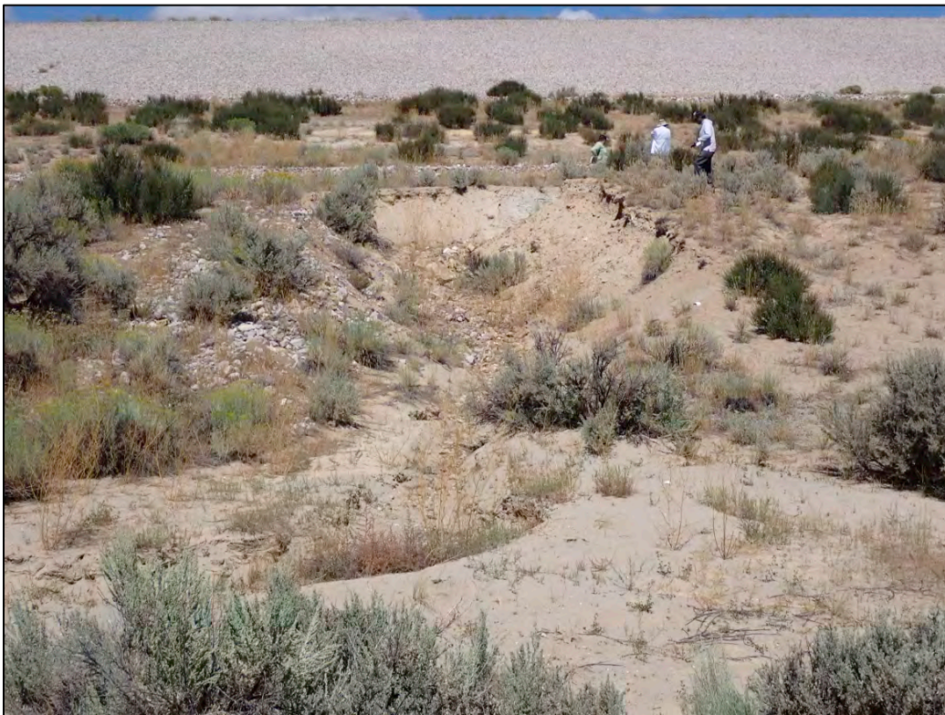
PL-14. Largest Gully Below Rock Berm
