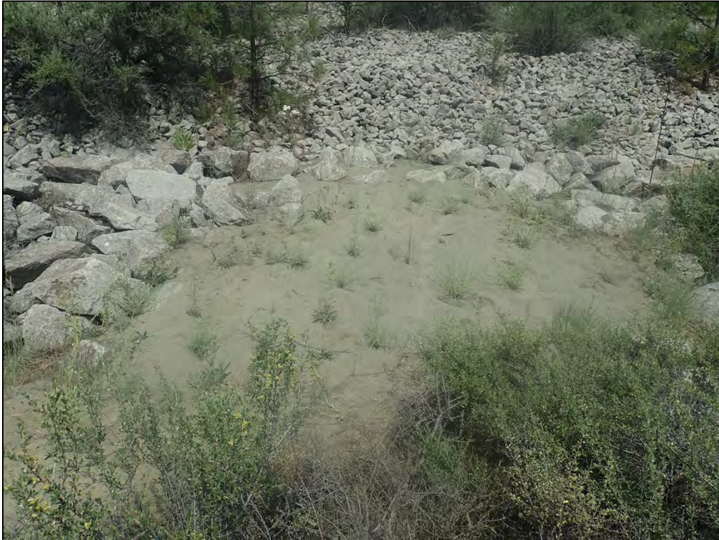
PL-9. Sand Deposit on Containment Dam
