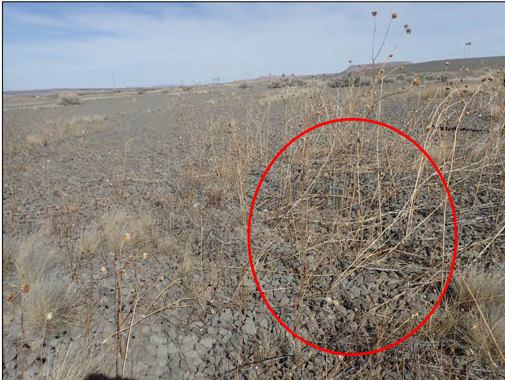
PL-21. Minor Depression with Vegetation Growth on Carbonate Tailings Disposal Cell Top Slope
