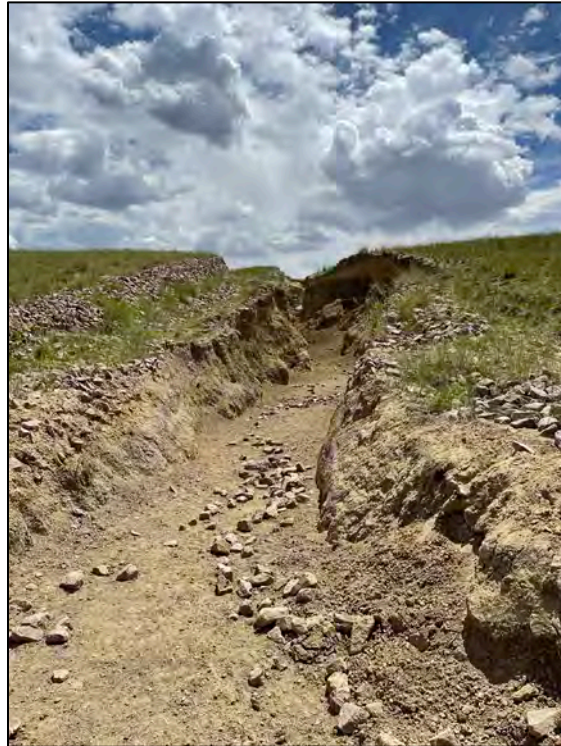
PL-16. Pit 4 Lower Riprap Armored Drainage Channel Erosion
