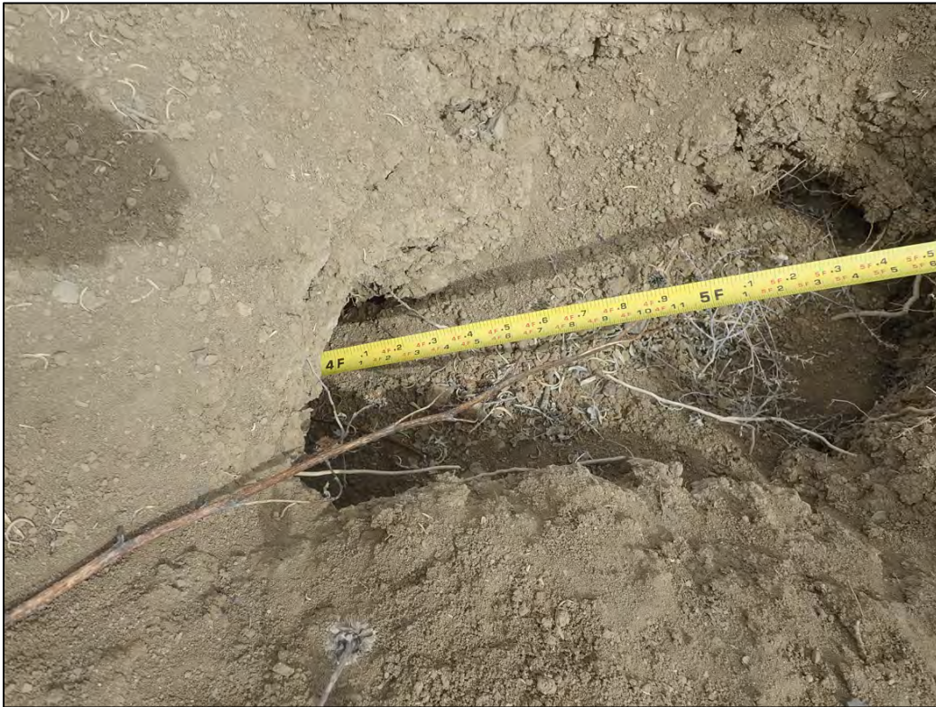
PL-11. Degradation Feature E-004 Horizontal Piping
