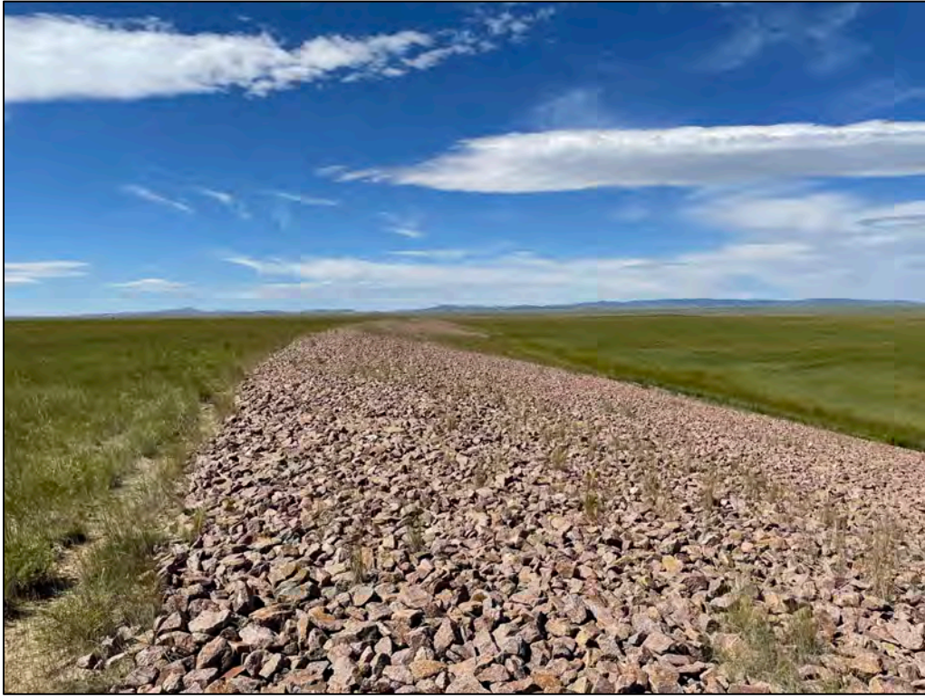
PL-9. Vegetation Encroachment on Upper Riprap Slope
