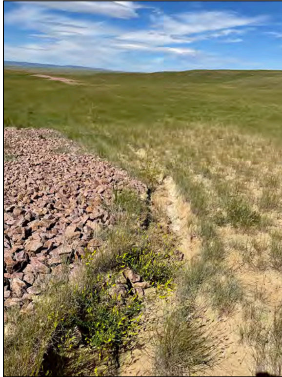
PL-7. Erosion Caused by Animal Trail North of Upper Riprap Slope
