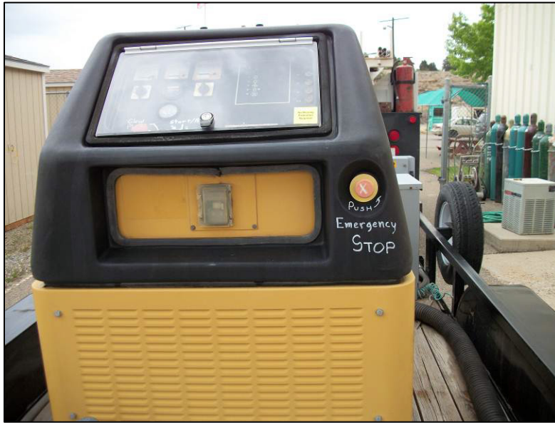
Figure 5. Emergency Stop Button
