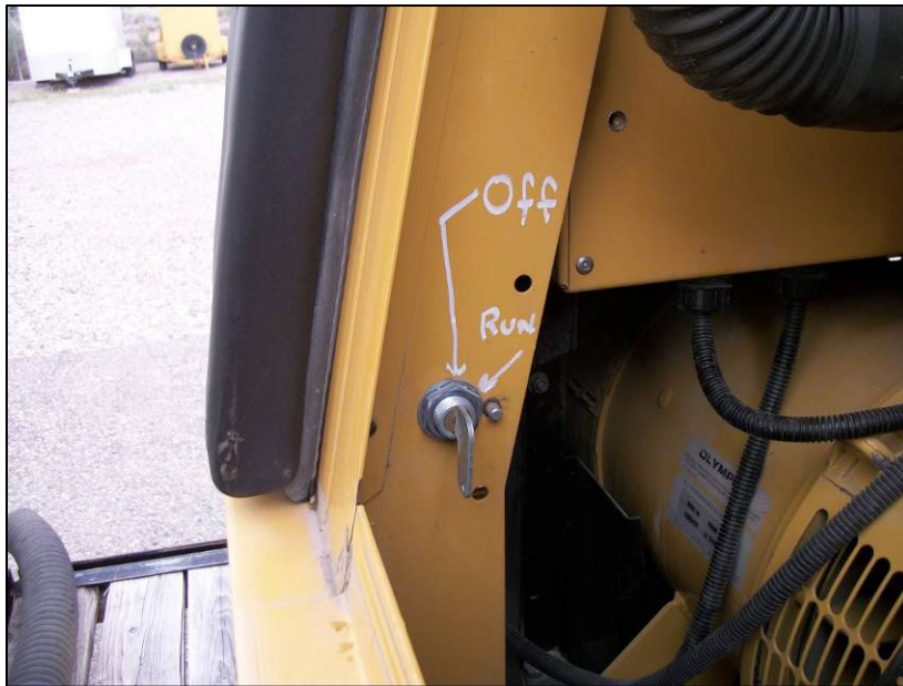
Figure 2. Battery Isolation Switch
