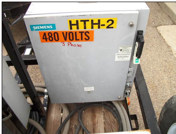
Figure 4. Typical Disconnect Switch
