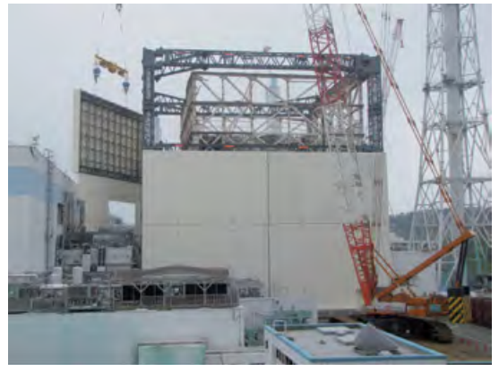
Figure 7-1 Enclosure for unit 1, view from the north 56
