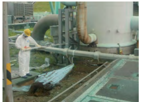
Figure 3-7 Base of stack between units 1 and 2, measurement with a telescopic detector 20
