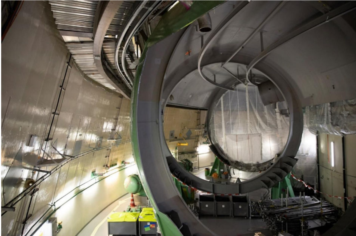
Figure 10: Reactor building – remaining support rings of the torus after completion of dismantling work Phase 1 (Photo BKW)
