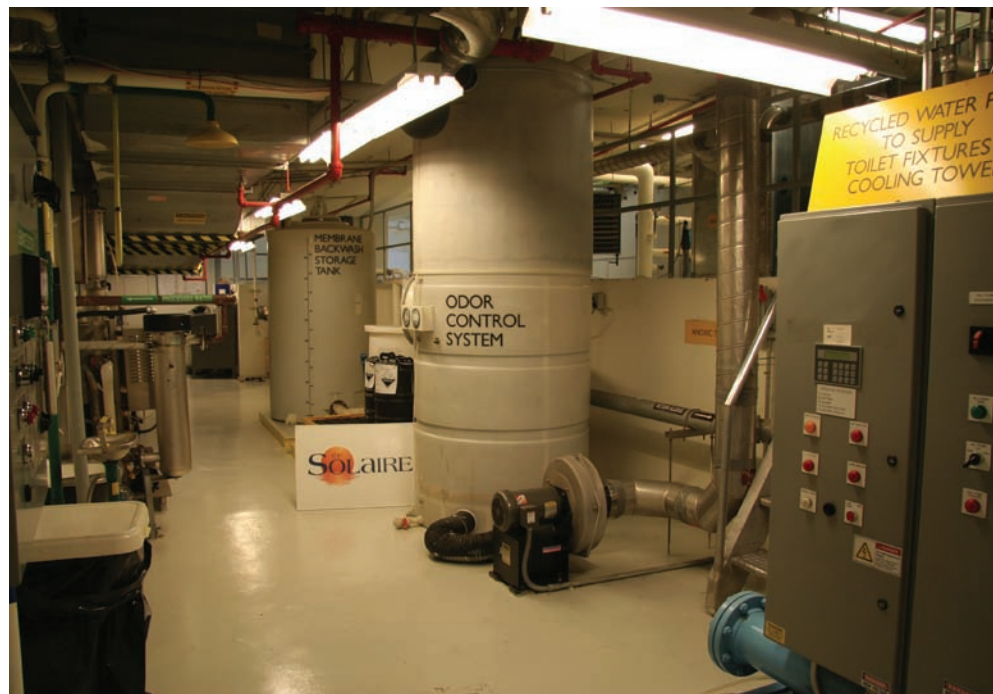
The Solaire's water treatment plant uses a process of digestion, membrane filtration and ultraviolet disinfection.
