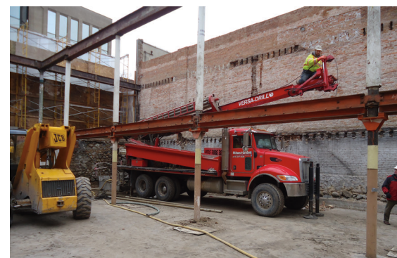
Maneuvering the drill rig into place for the first bore holes to be drilled.
