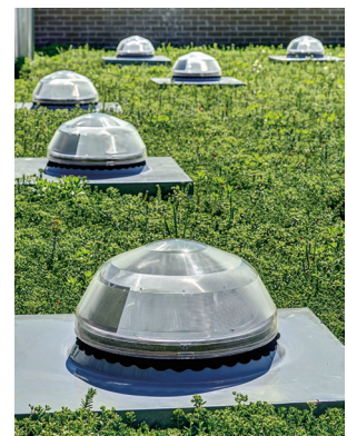
Solar light tubes on the vegetative roof provide natural light deep into the building.
