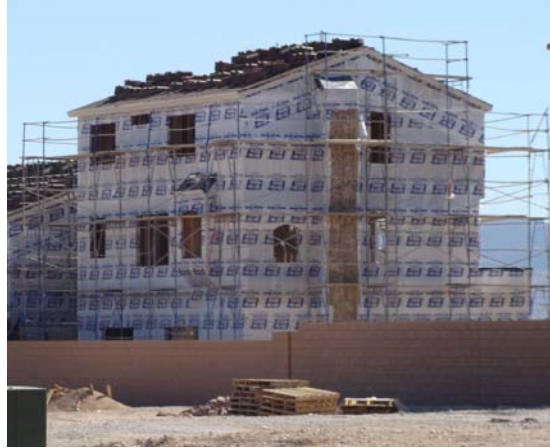
Figure 28 - Welded end frame scaffold.
