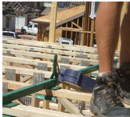
Figure 17 - A retractable lifeline attached to a floor truss anchor.
