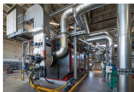
Figure 5. Hot-water boiler “BOSCH UT M-64”.
