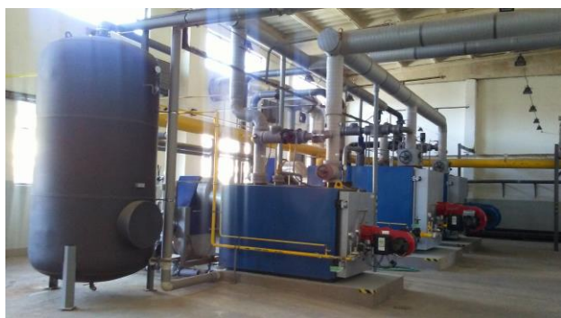
Figure 2. Interior view of the existing boiler plant [7]
