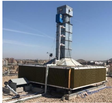
Figure 1. Experimental facility located in ELDI building, Technical University of Cartagena (Spain).
