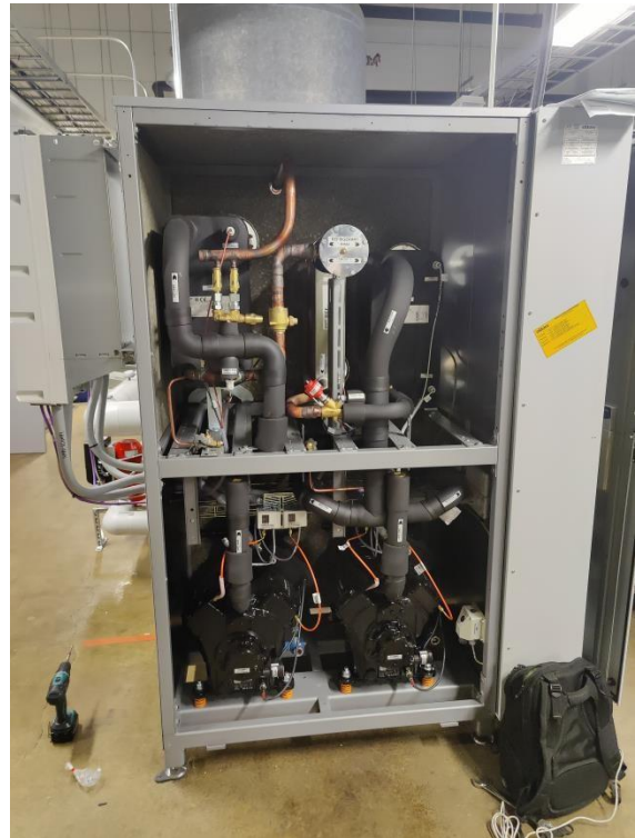
Figure 2. Heat pump operating as an energy recycling heat pump in a hybrid heating system.
