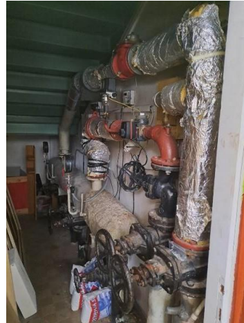
Figure 2 Heat transfer station of Kindergarten
